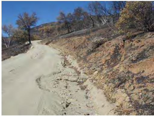
Picture 18 Heavily Damaged Road Leading to Water Tanks
