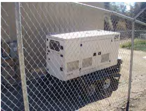
Picture 16 Generator Used to Power Water Lines
