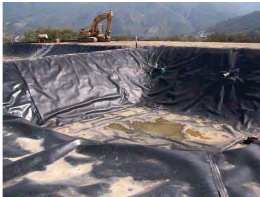
Picture 14 Wastewater Treatment Plant
